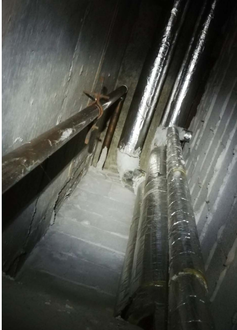
Photo 1: Inaccessible Exposed Parging on Pipe Elbow
