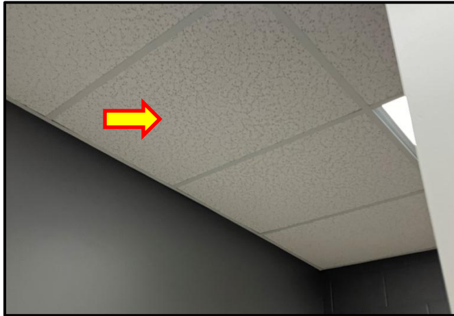
Photograph 5: View of non-asbestos containing 2'x4' acoustic ceiling tiles observed throughout the building.
