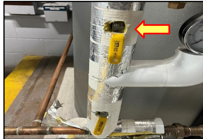
Photograph 4: View of non-asbestos containing fiberglass insulation observed on mechanical pipe fittings throughout.
