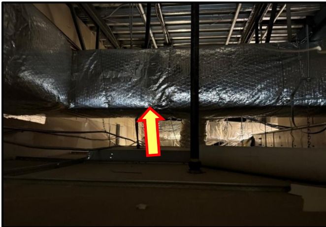
Photograph 7:View of the non-asbestos fiberglass insulation observed on ductwork within ceiling spaces.
