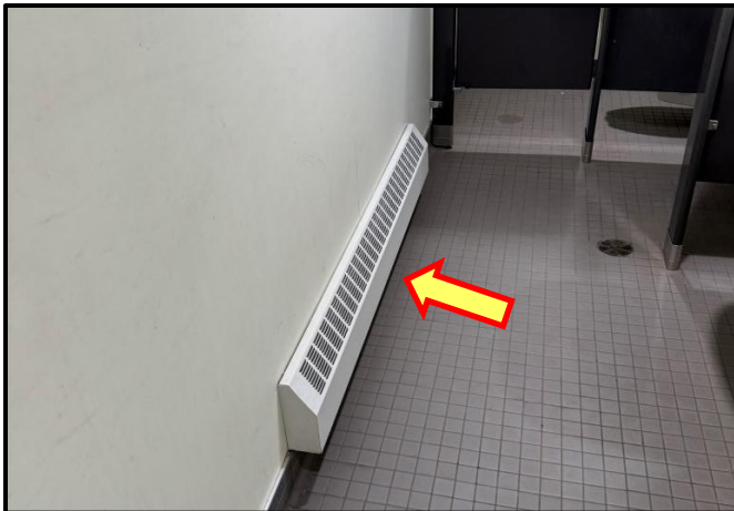
Photograph 3: Typical view of the baseboard heaters observed throughout the building.
