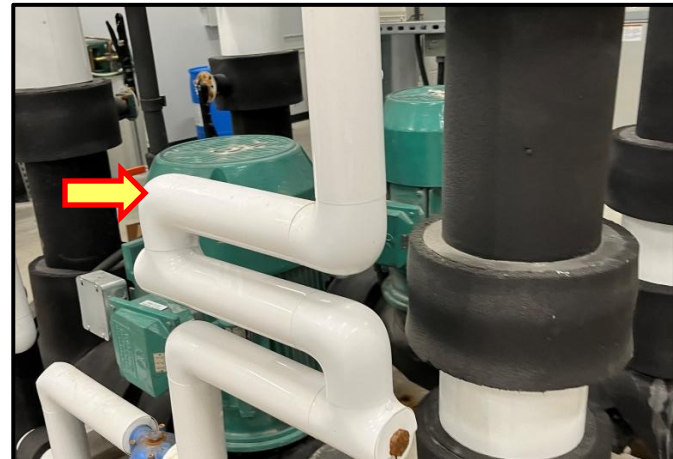
Photograph 4: View of non-asbestos containing fiberglass insulation with PVC cover on mechanical pipes observed.
