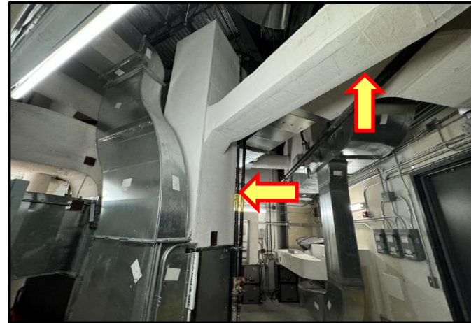
Photograph 6: View of non-asbestos fiberglass insulation observed on ductwork in the mechanical room (E202).
