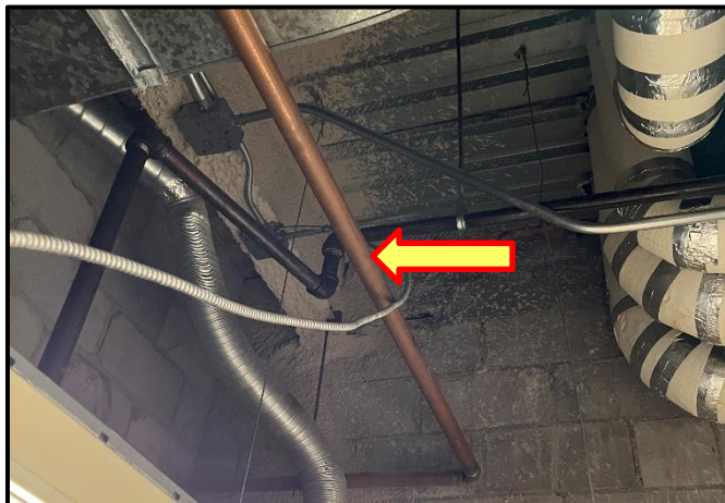
Photograph 13: View of potentially lead-containing copper piping observed throughout the building in ceiling spaces.
