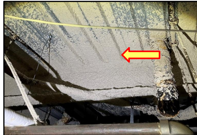
Photograph 8: View of non-asbestos containing sprayed fireproofing observed in ceiling spaces throughout the building.
