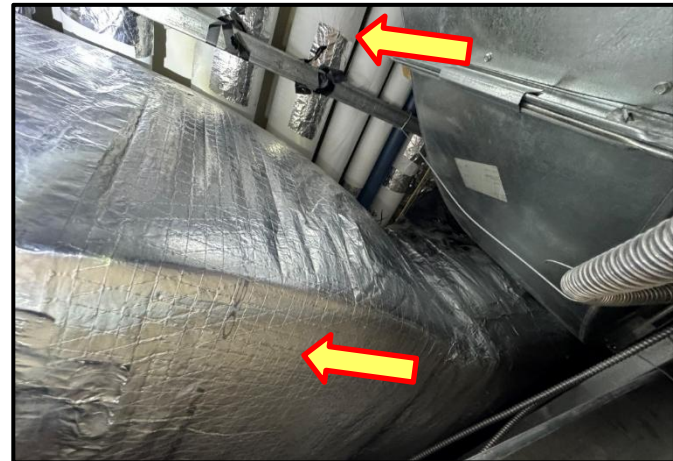
Photograph 8:View of fiberglass insulation observed on ductwork and mechanical pipes in ceiling spaces throughout Building A.
