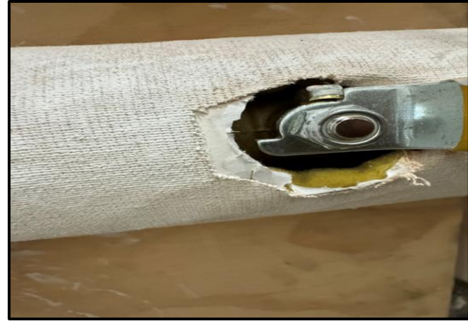
Photograph 2:View of mechanical pipes insulated with non-asbestos applications of fiberglass.
