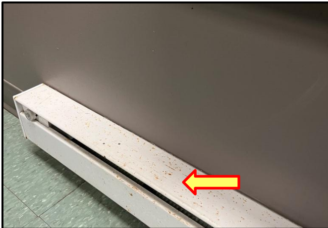
Photograph 7: View of electric baseboard heaters observed throughout the building.
