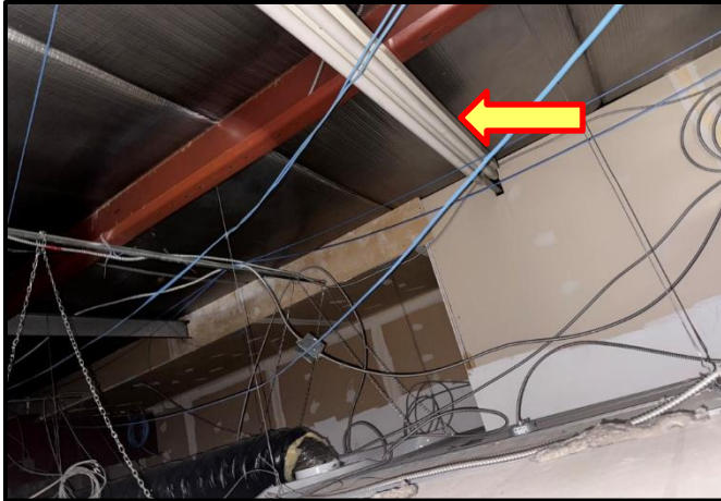
Photograph 9: View of potentially mercury containing fluorescent lighting observed above the suspended grid ceiling in Room 201.
