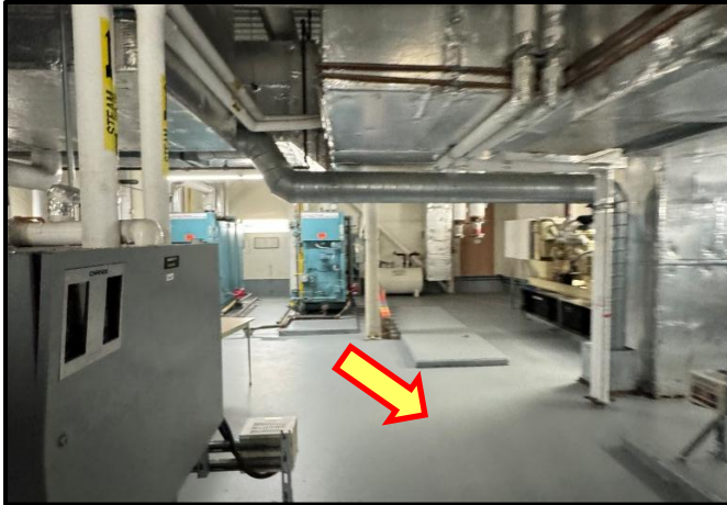
Photograph 9: View of lead-containing grey paint observed in the Chiller Plant Area (Room J400) .
