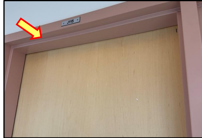
Photograph 10: View of lead-containing pink door frame paint observed throughout the building.
