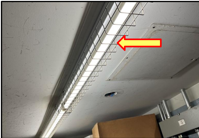
Photograph 3: View of potentially mercury containing fluorescent lighting observed throughout the building.
