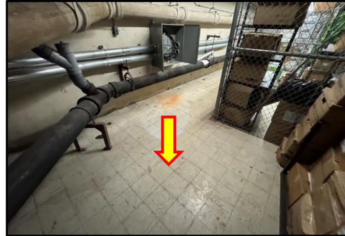
Photograph 2: View of asbestos-containing 9"x9" beige vinyl floor tiles observed in the basement corridor.
