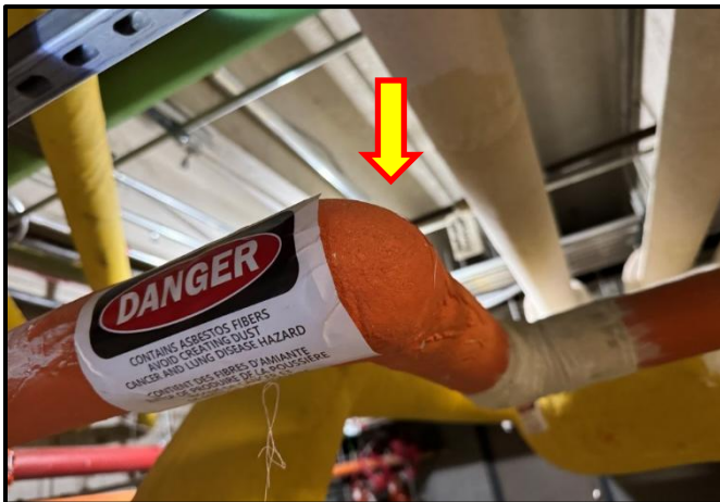
Photograph 3: View of asbestos-containing paring cement mechanical pipe elbow fittings observed throughout the basement tunnels.
