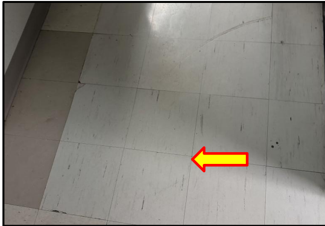
Photograph 9:View of asbestos-containing grey 12"x12" vinyl floor tiles observed in Room A1451c.
