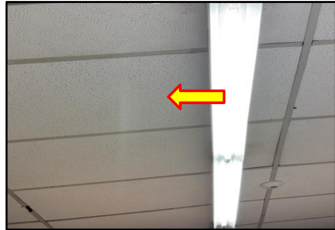
Photograph 10:View of asbestos-containing 2'x4' acoustic ceiling tiles observed in Room A1207.
