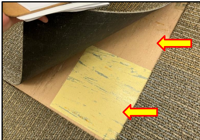
Photograph 7: View of asbestos-containing light brown and yellow 9"x9" vinyl floor tiles observed under carpet tiles in Room A2127.
