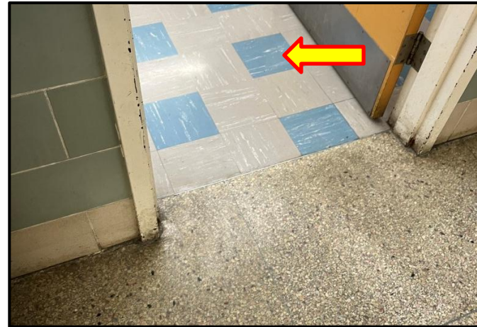
Photograph 6: View of asbestos-containing light blue and grey 9"x9" vinyl floor tiles observed in Room A2113.
