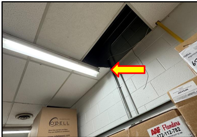
Photograph 11: View of damaged asbestos-containing 2'x4' acoustic ceiling tile observed in Room A1207.
