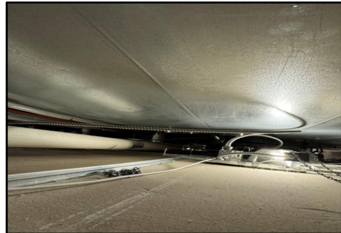
Photograph 4: View of mechanical pipes insulated with non-asbestos fiberglass within the ceiling spaces.
