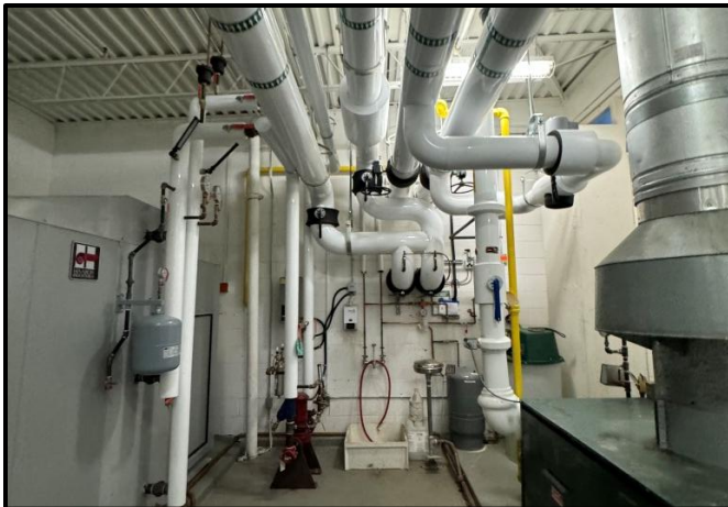
Photograph 3: View of mechanical pipes insulated with fiberglass and PVC located in the second-floor mechanical room.
