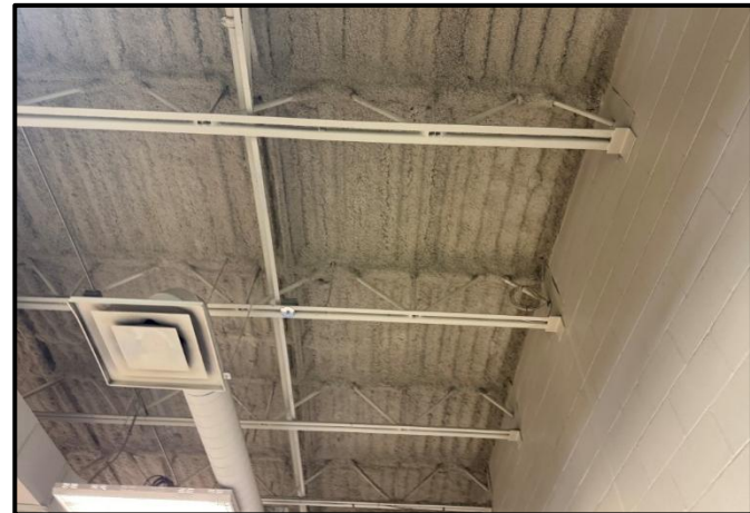
Photograph 8: Typical view of sprayed on fireproofing observed in ceiling spaces throughout the building.
