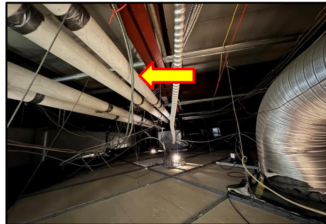
Photograph 8: View of asbestos-containing aircell pipe insulation observed on mechanical pipe straight runs in the ceiling of Room D101D.
