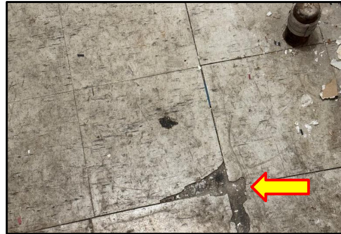
Photograph 2: View of damaged asbestos-containing 12"x12" beige vinyl floor tiles with black streaks observed in Room D117.
