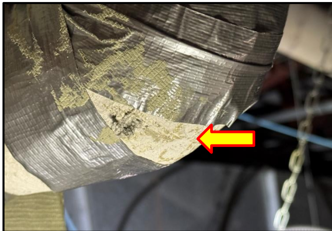
Photograph 7: View of damaged asbestos-containing paring cement mechanical pipe fitting observed in the ceiling space of Room D101D.
