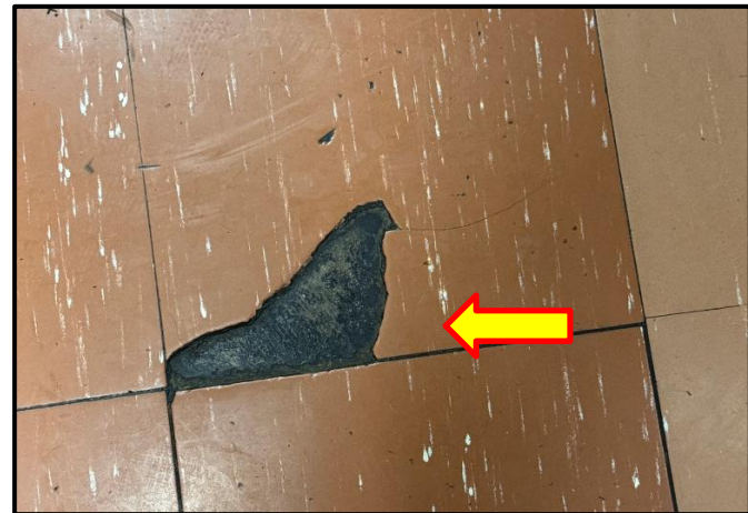
Photograph 4: View of damaged asbestos-containing 12"x12" red vinyl flooring tiles observed in Room D108.
