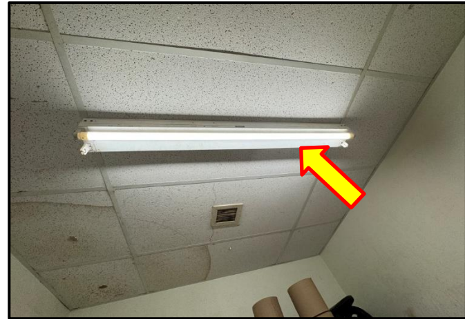
Photograph 6: Typical view of mercury containing fluorescent lighting observed throughout the building.
