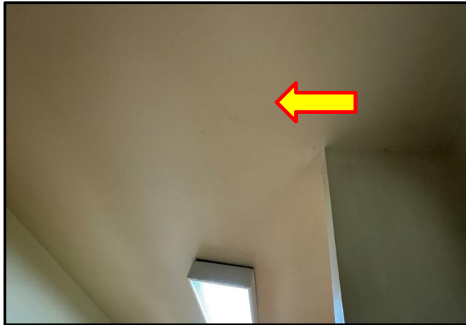
Photograph 5: View of asbestos-containing ceiling plaster observed in Room D106.
