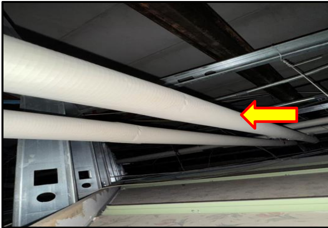
Photograph 9:View of non-asbestos containing fiberglass insulation observed on mechanical pipe straight runs throughout the building.
