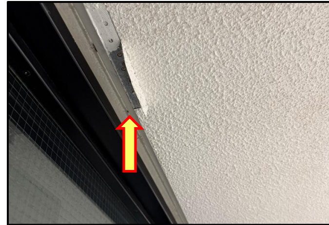
Photograph 14:View of damaged asbestos-containing ceiling stipple observed in the corridor outside Room B115B.
