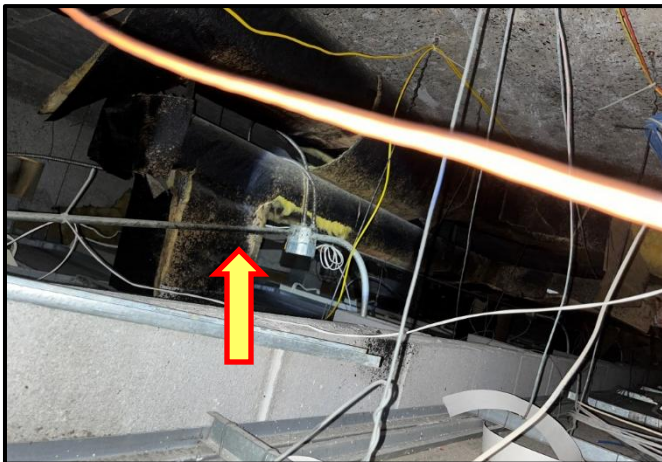
Photograph 7: View of asbestos-containing black tar in poor condition observed on ductwork in the ceiling space of Room B311A.
