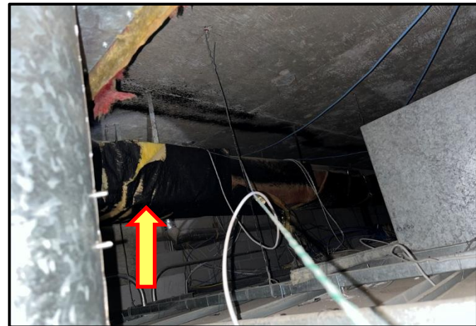
Photograph 8: View of asbestos-containing black tar in poor condition observed on ductwork in the ceiling space of Room B302.
