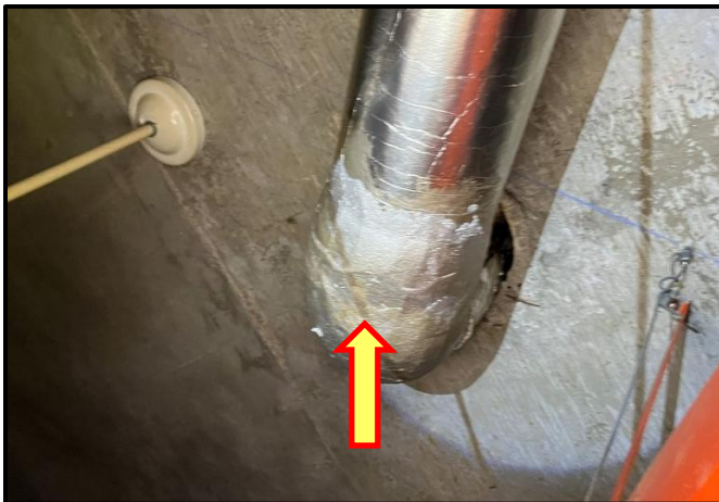
Photograph 11: View of asbestos-containing silver pipe elbow fitting observed in the ceiling space of Room B419.
