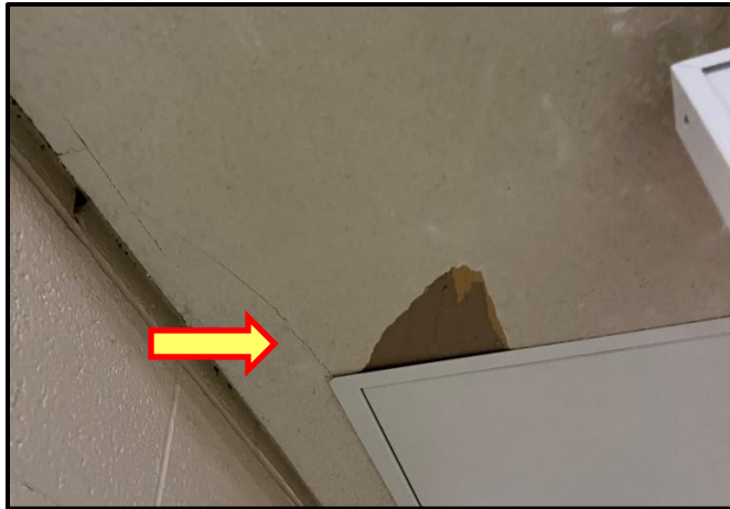
Photograph 13:View of asbestos-containing ceiling stipple observed in poor condition in the corridor outside Room B443.
