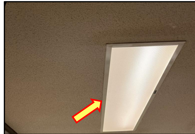
Photograph 16:Typical view of mercury containing fluorescent lighting observed throughout the building.
