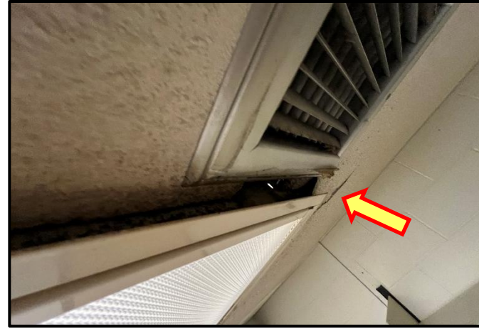
Photograph 18:View of asbestos-containing ceiling stipple observed in poor condition in the corridor outside Room B439.
