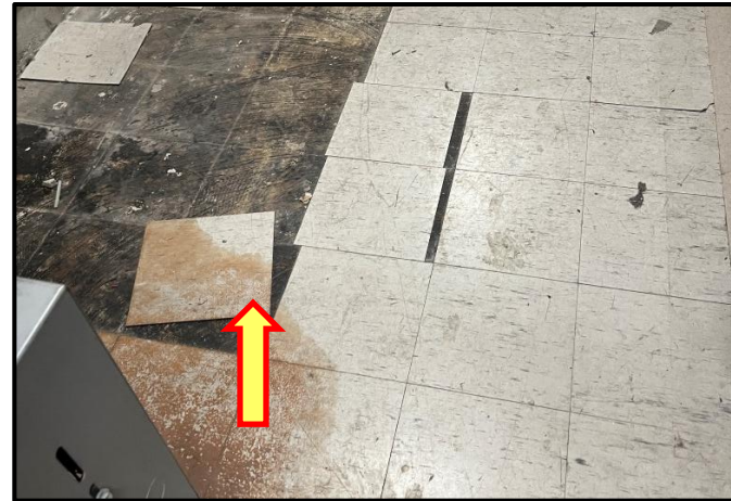
Photograph 6: View of asbestos-containing 12"x12" Grey vinyl floor tiles in poor in Room B362.
