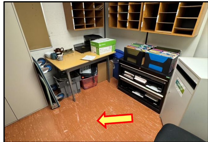
Photograph 4: View of asbestos-containing 12"x12" red/orange vinyl floor tiles observed in Room B136S.
