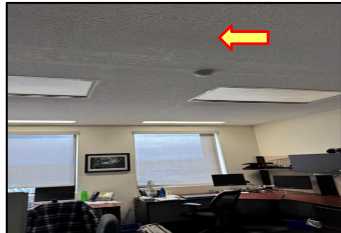
Photograph 12:View of asbestos-containing ceiling stipple observed in Room C530.
