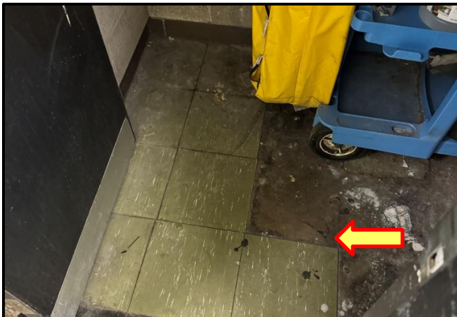
Photograph 3: View of damaged asbestos-containing green 12"x12" vinyl floor tiles observed in Room C232.
