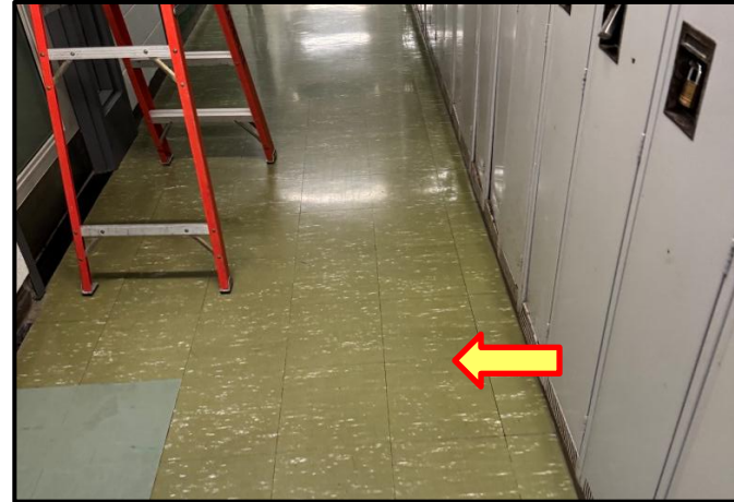
Photograph 2: View of asbestos-containing green 12"x12" vinyl floor tiles observed in the second-floor corridor.
