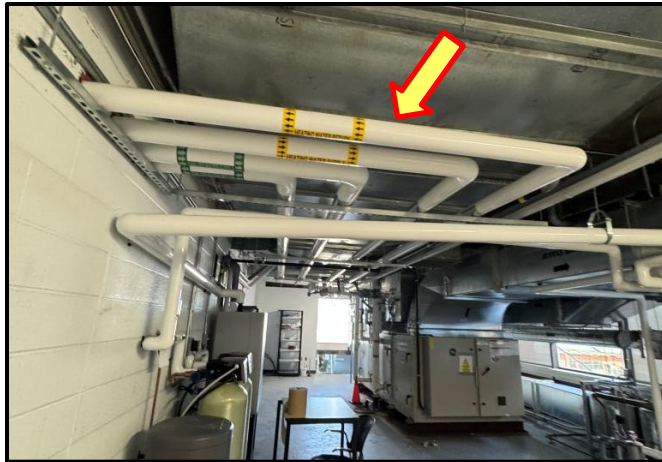
Photograph 9:View of the non-asbestos containing fiberglass and PVC pipe insulation observed in Room C341.
