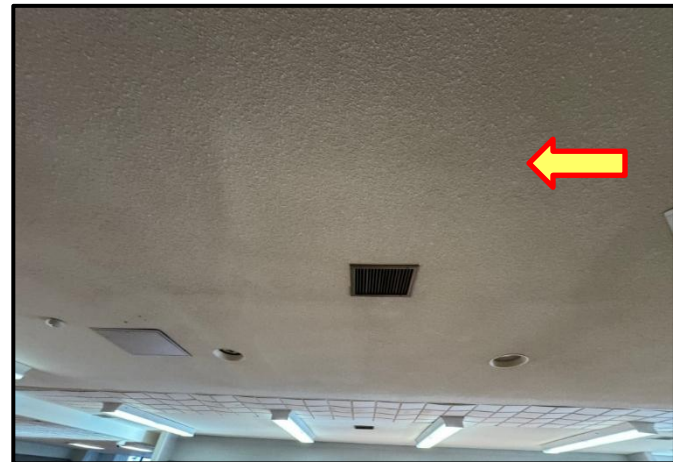
Photograph 8: View of asbestos-containing ceiling stipple observed in Room C348.
