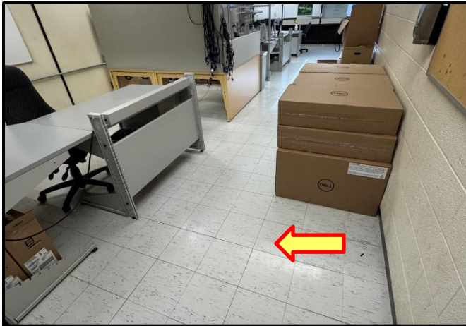
Photograph 5: View of the asbestos-containing grey 12"x12" vinyl floor tiles observed in Room C340.
