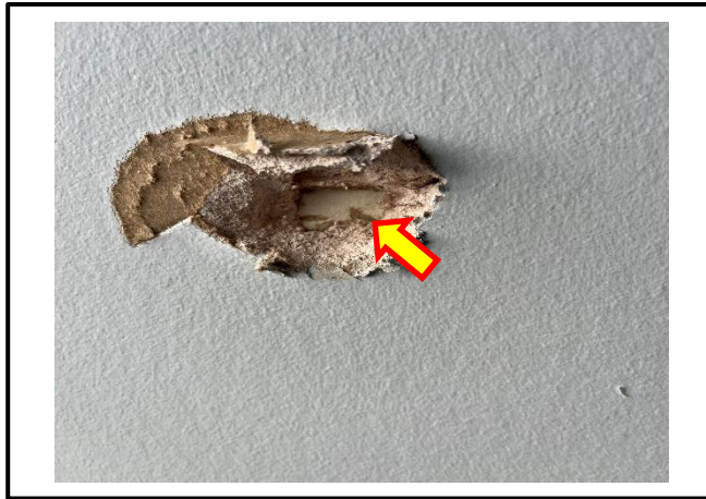
Photograph 5: View of the presumed asbestos-containing drywall observed under non-asbestos drywall throughout the building.
