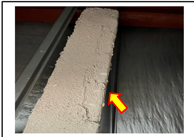
Photograph 3: View of the asbestos-containing textured plaster (Fireproofing) observed on structural beams throughout the building.
