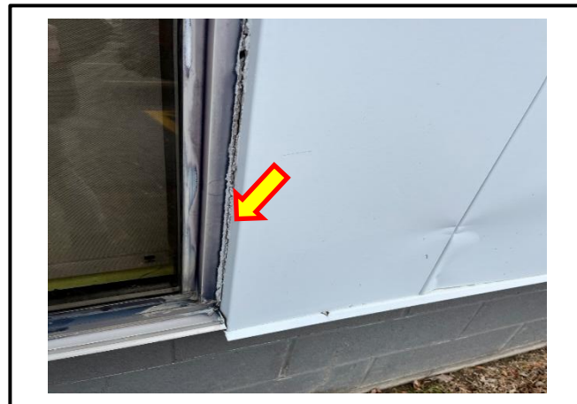
Photograph 4: View the asbestos-containing exterior window caulking observed on the exterior windows throughout the building.
