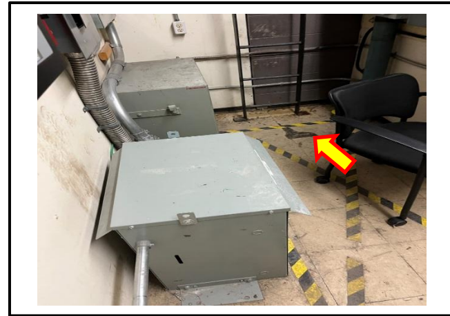
Photograph 2: View of the damaged asbestos-containing beige vinyl floor tiles observed in Electrical Room F113b.
