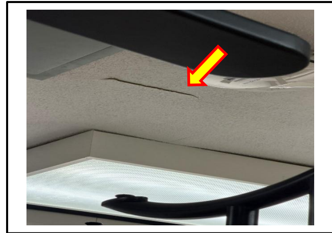
Photograph 6: View of the damaged/delaminating asbestos-containing ceiling stipple observed in Room 215B.
