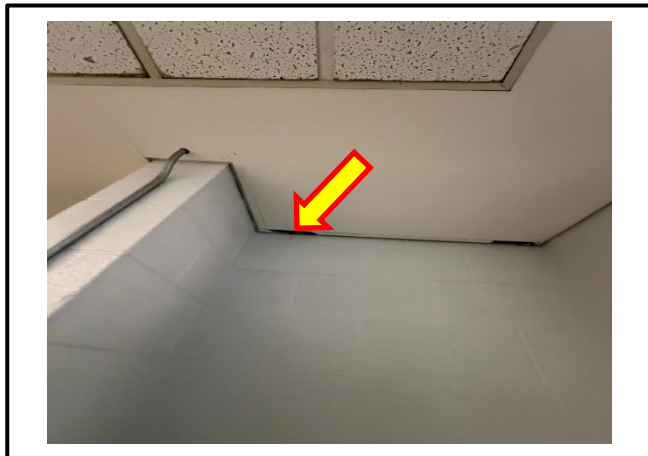
Photograph 7: View of the damaged asbestos-containing drywall joint compound observed
