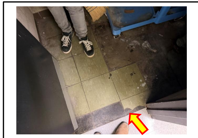
Photograph 4: View of damaged 12"x12" green vinyl floor tiles observed in Room C232.
