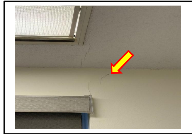
Photograph 10: View of the damaged asbestos-containing drywall joint compound observed in Room C530.
