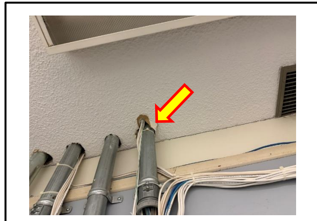
Photograph 8: Typical view of the damaged asbestos-containing ceiling stipple observed throughout the fourth-floor corridor.
