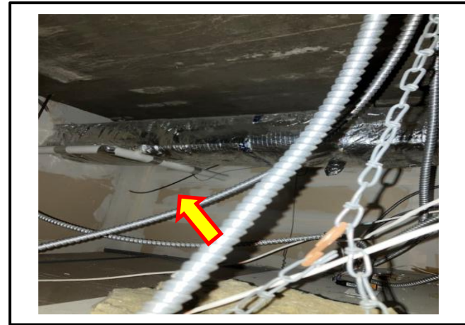
Photograph 2: View of the asbestos-containing drywall joint compound observed above the ceiling space in the first-floor clinic.
