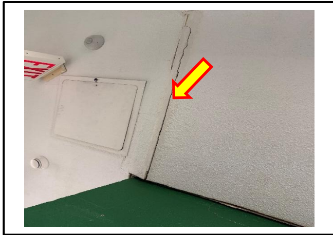
Photograph 9: Typical view of the damaged asbestos-containing ceiling stipple observed throughout the fifth-floor corridors.
