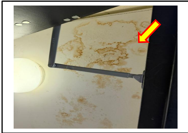
Photograph 5: View of the damaged/moisture-stained drywall joint compound on the ceiling in Room C231.
