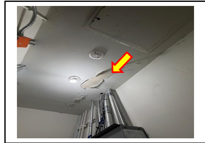
Photograph 6: View of the damaged asbestos-containing drywall joint compound on the ceiling of Room D117.
