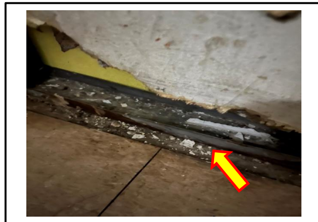
Photograph 4: View damaged asbestos –containing drywall and debris observed in the stairwell leading to the second-floor mechanical room.
