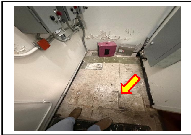
Photograph 5: View of the damaged asbestos-containing 12"x12" beige vinyl floor tiles with black streaks observed in Room D117.
