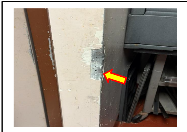
Photograph 7: Typical view of the damaged asbestos-containing drywall joint compound on walls and corner beads throughout Room D119.
