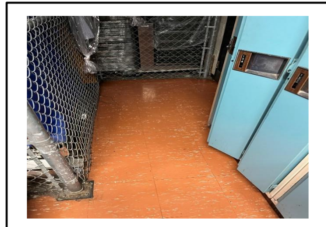
Photograph 8: Typical view of the asbestos-containing 12"x12" red vinyl floor tiles observed in Room D108.
