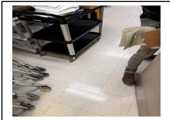
Photograph 7: View of the asbestos-containing 12"x12" white vinyl floor tiles with black and grey streaks observed in Room A2114.
