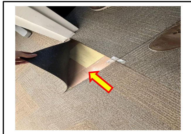
Photograph 8: View of the asbestos-containing 9"x9" vinyl floor tiles observed under carpet in Room A2127.
