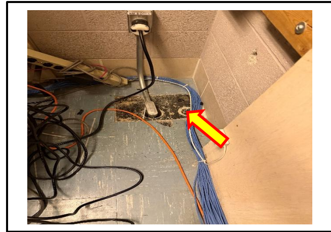
Photograph 2: View of the damaged asbestos-containing 9"x9" blue vinyl floor tiles and exposed asbestos-containing mastic observed in Room A1208A.
