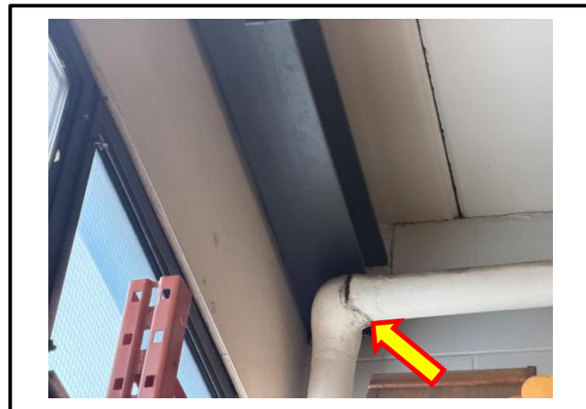
Photograph 4: View of the damaged asbestos-containing parging cement pipe elbow fitting observed in Room A1445.
