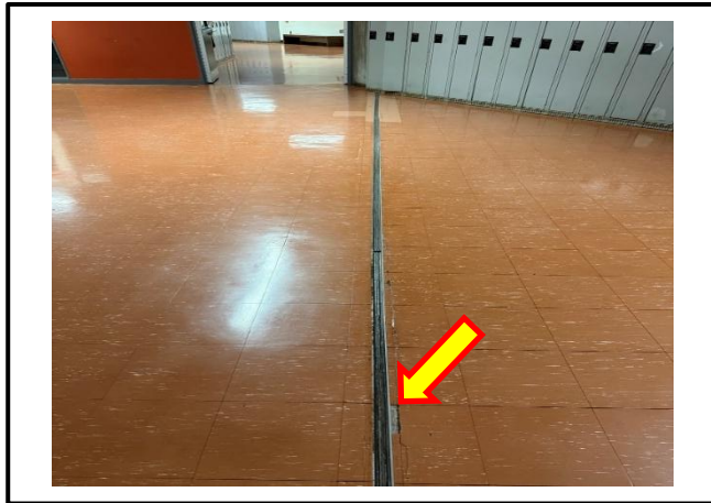
Photograph 9: View of the damaged asbestos-containing 12"x12" red/orange vinyl floor tiles observed in the third-floor corridor outside Room B355.
