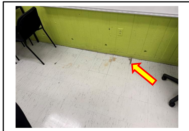
Photograph 4: View of the damaged asbestos-containing 12"x12" white/grey vinyl floor tiles observed in Room B133.
