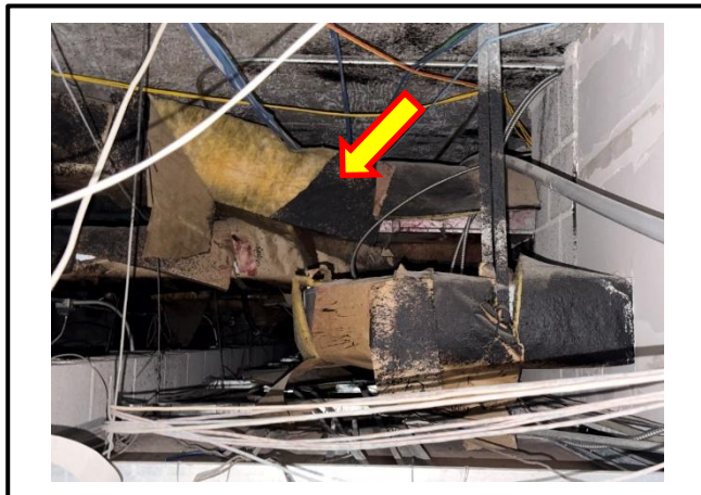
Photograph 11: View of the damaged asbestos-containing black tar on ductwork in the ceiling space in the corridor outside Room B311A.
