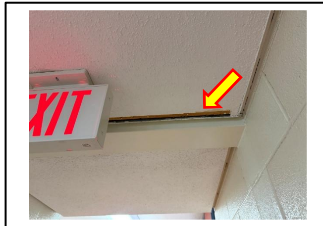
Photograph 8: Typical view of the damaged asbestos-containing ceiling stipple observed in the third-floor corridors.
