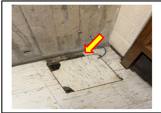
Photograph 5: View of the damaged asbestos-containing 12"x12" grey vinyl floor tiles observed in Room B137A.
