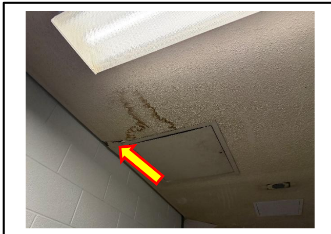
Photograph 3: View of damaged asbestos-containing ceiling stipple in the corridor outside Room B170.
