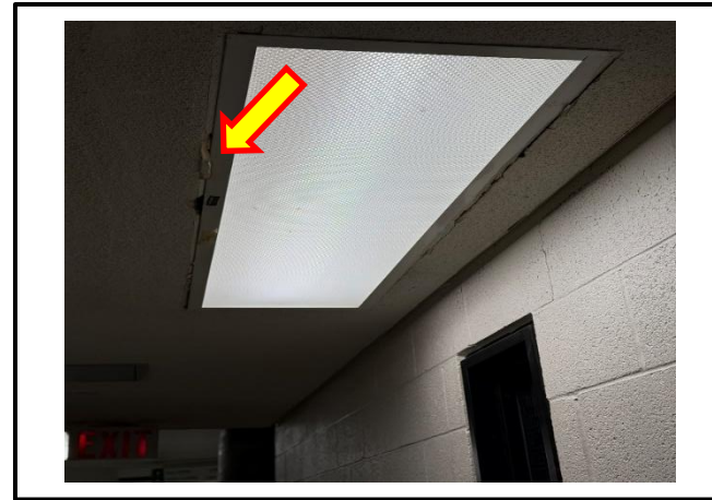
Photograph 6: View of the damaged asbestos-containing ceiling stipple observed on light fixtures throughout the second-floor.
