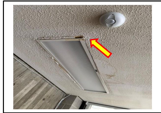
Photograph 2: View of the damaged asbestos-containing ceiling stipple observed around light fixtures in Room B146.
