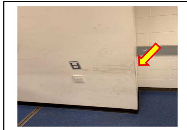
Photograph 12: View of the damaged asbestos-containing drywall joint compound observed in Room B383.
